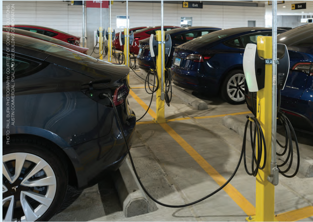
The new facility is slated to have 60 charging stations by the end of this year.
